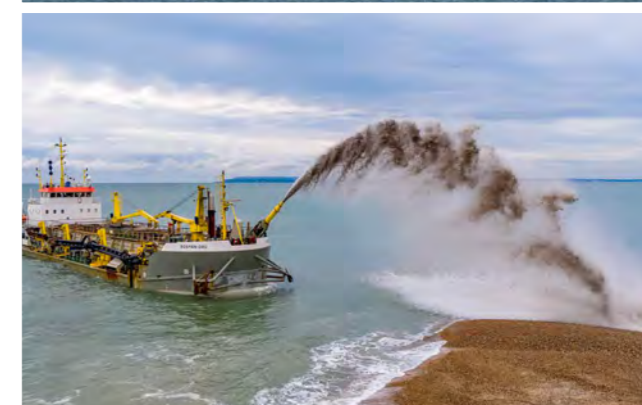
Figure 2.2: Different disposal techniques, from top: Clam shell excavation from hopper (Carol Reid); release of hydraulically pumped sediment via pipeline (Exo Environmental Ltd.); spud barge and hopper barge at marsh transfer and hydraulic pumping station (ABPmer); and coarse sediment rainbow discharge (Boskalis).
