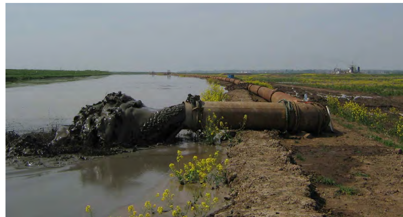
Figure 2.9: Hydraulic disposal by pipeline and the last disposal of 550,000m 3 of fine sediment prior to breaching of the flood defences at Allfleet's Marsh, Crouch Estuary, Essex (ABPmer).
