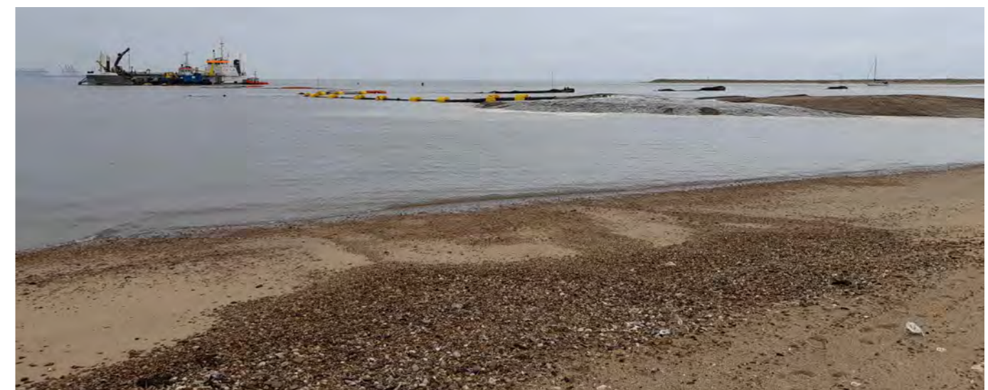
The most recent works undertaken at the Horsey Island site (October 2021). A trailing suction hopper dredger was used to recharge the barrier with sand and gravels arising from the deepening of the Harwich and Felixstowe approach channel. Approximately 10,000 m 3 of the total 50,000 m 3 being used during the project can be seen on the right shortly after disposal. The sediment was hydraulically pumped via floating pipeline and will allow natural processes to redistribute the material along the coast. These works were undertaken through a partnership between the local landowner, the RSPB, Harwich Haven Authority and the Environment Agency (Will Manning, Cefas).
